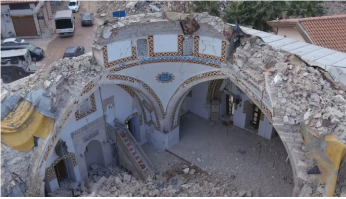
Figure 1- Destruction in Habibi Neccar Mosque 1
