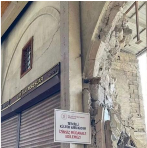
Figure 6- Damaged cultural property sign (Architect Birsen Parlar archive)
